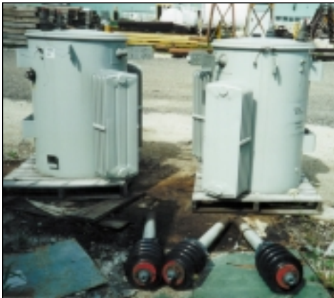
Transformer Storage Yard – Ying-Kuang Hsu
