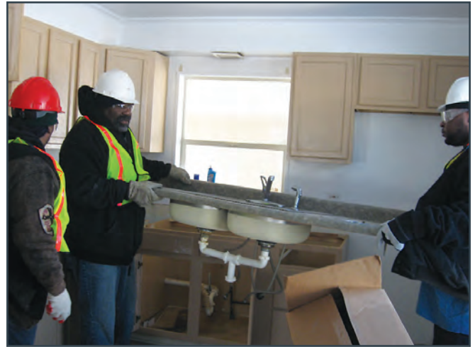
Trainees remove a sink during a deconstruction course taught by Delta Institute and RE-USE Consulting, Inc. (Photo by Delta Institute.)
