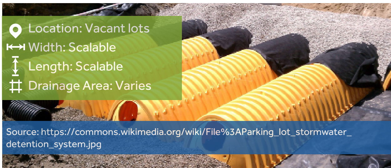
Figure 10: Underground storage chambers for stormwater
